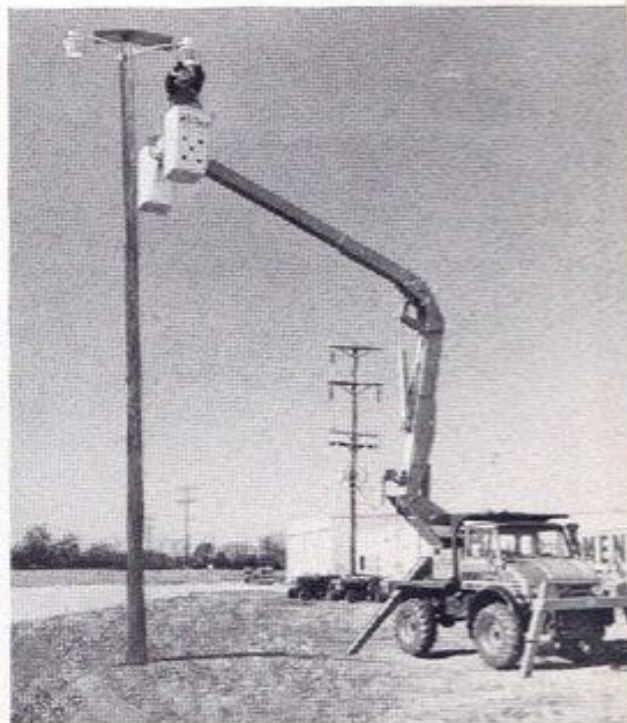
Unimog rises to the occasion with this twin manbasket. Utility personnel have a working height of 45', with 360° rotating capability which can be controlled from either manbasket or from the ground.
